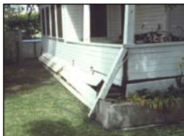
Figure 12: Damage caused by unbraced cripple walls. Note that the house has shifted about 1 foot (30 cm) off its foundation (WHE Report 90, USA)
