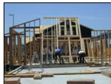
Figure 6: Installation of prebuilt stud wall on reinforced concrete floor slab (WHE Report 90)
