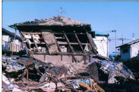
Figure 14: Damage caused by heavy roof construction in Japan from 1995 Kobe earthquake (WHE Report 86)
