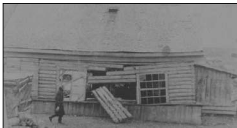
Figure 11: A photograph illustrating typical earthquake damage from the 1958 Kamchatka earthquake (WHE Report 56)
