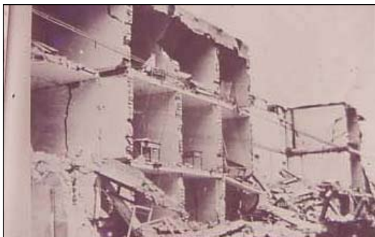
Figure 8: Typical earthquake damage to brick masonry buildings without base isolation (1976 Tanshan earthquake) (WHE Report 9, China)
